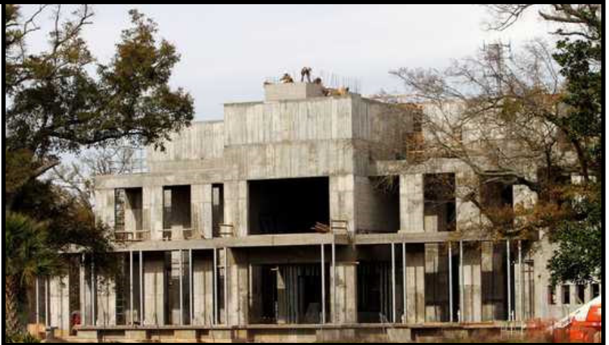
JOHN FITZHUGH/SUN HERALD The Jefferson Davis Presidential Library and museums under construction at Beauvoir in Biloxi
